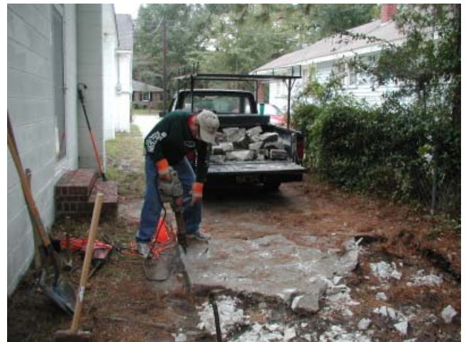
Driveway repair in progress Member BJ Smith breaking concrete with his jack hammer
